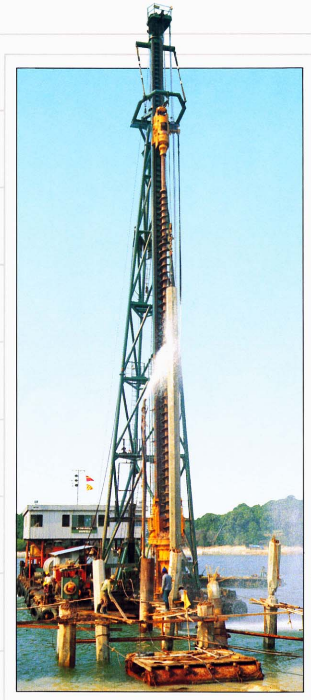
SDA-180KWP on a pontoon in Singapore Refer to Page 8.
